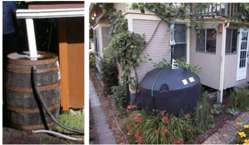
Rain Barrel and Tank Example
